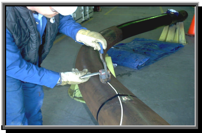
Figure 1-1. A trainee fastens a lead wire to a steel pipe with a thermite weld(er).
