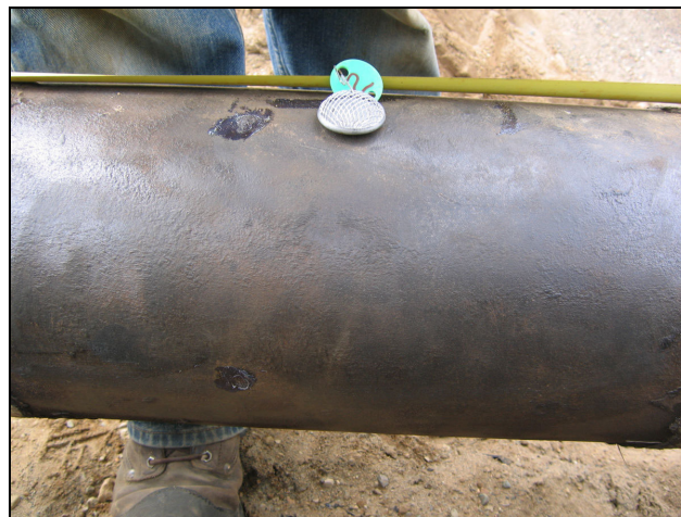
FIGURE 11 • DE #2 • Pipe Exposed. Close View.
