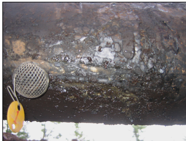
FIGURE 15 • DE #1. Coating Damage. 20 cm x 5 cm Holiday #1.
