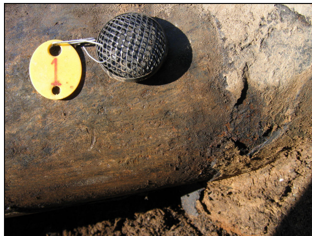
FIGURE 5 • Site #1. Pipe Exposed. Close View at Holiday #1
