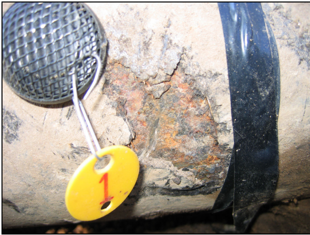
FIGURE 3 • Site #1. Coating Damage. 4 cm Dia. Holiday #1
