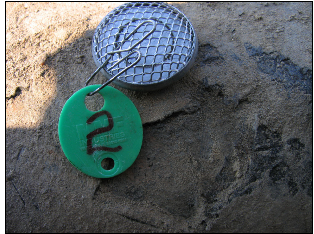
FIGURE 4 • Site #1. Coating Damage. 3 cm Dia. Holiday #2
