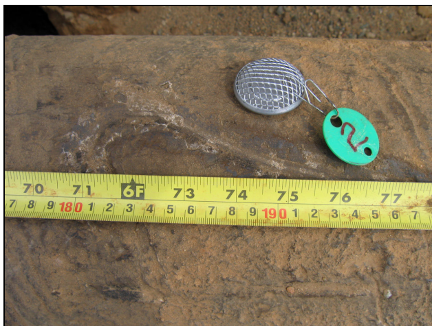
FIGURE 8 • DE #2. Coating Damage. Holiday #1 (Tag #2).
