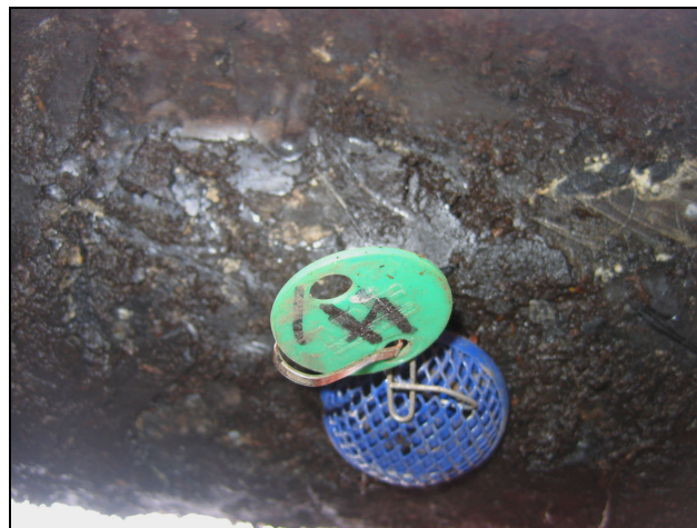
FIGURE 17 • DE #2. Coating Damage. 5 cm Dia. Holiday #4.
