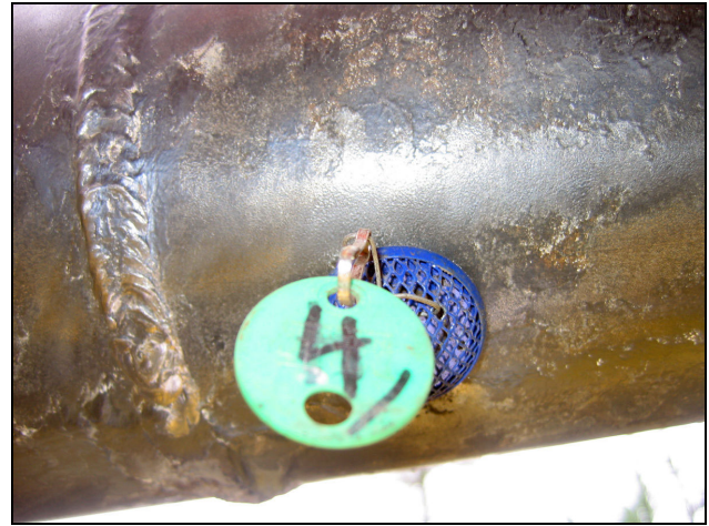
FIGURE 19 • DE #2 Pipe Exposed at Holiday #4. Close View.
