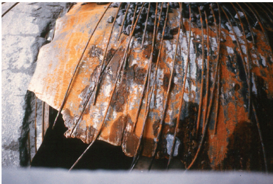
Typical corrosion failure of a prestressed concrete cylinder pipe.
