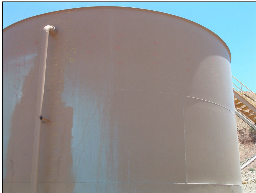
Photo 1. Sulphuric acid tank containing NOX contaminated acid. Ultrasonic measurements revealed accelerated corrosion.
