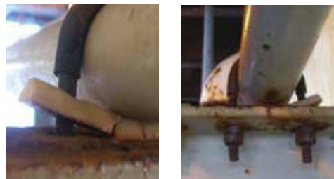
Failed I-Rod® imitations.
