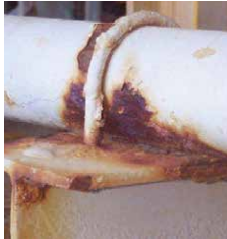
Above, the result of crevice corrosion on a pipe. Trapped moisture has caused substantial wall loss that could result in catastrophic failure.
