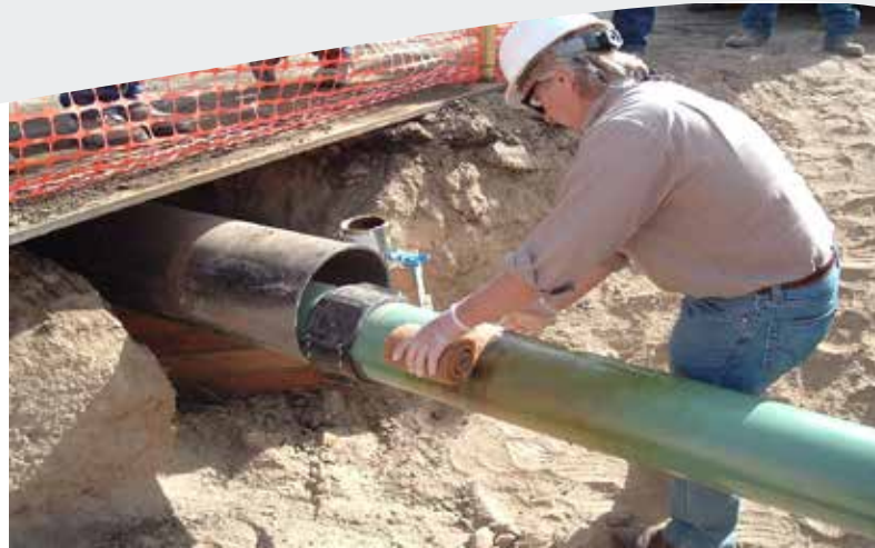
Wax-Tape HT-3000 wrap does not require sandblasting. Here the wrap is being applied to moderate-temperature pipe, but it can also be applied to hot in-service lines by using insulated gloves.
