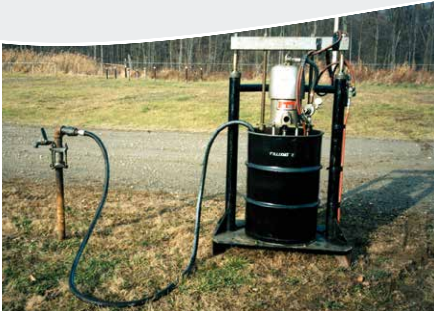
Fill-Coat #2 being pumped by air-driven mastic pump from 55-gallon drums into the casing vent.
