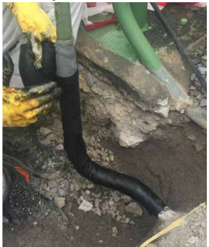
For irregularly shaped pipe or fittings, MCO 110 outerwrap has good conformability. The transition here shows how MCO 110 wrapped over Wax-Tape ® #2 anticorrosion wrap will provide excellent protection against frost heave and possible mechanical damage.
