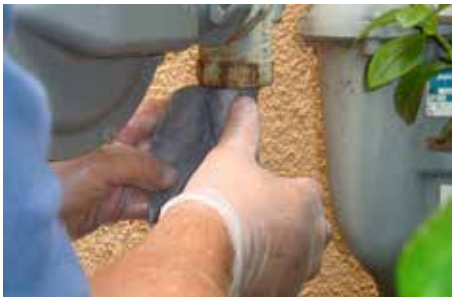
7. Starting at the bottom of the riser, firmly press the Wax-Tape® wrap around the pipe with the seam facing toward the back of the pipe. When using additional pads, use a minimum of 1" overlap.
