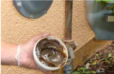
4. Hand apply the primer. Firmly rub and press the primer onto the surface to displace the moisture and ensure that the primer is adhering to the metal surface.
