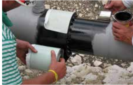
First layer of Double-Faced Adhesive is applied to the casing, Seal-Wrap Primer being applied to the carrier.
