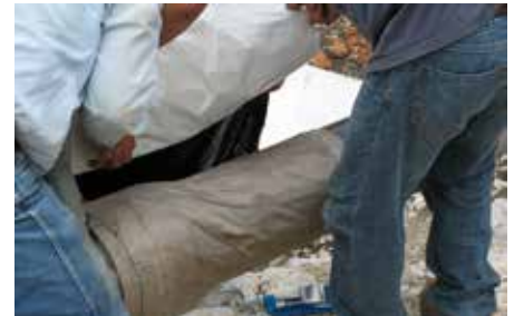
A second continuous wrap of Seal-Wrap applied directly over the first wrap.
