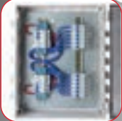
9. DC surge protection
